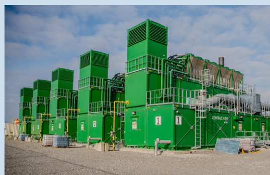
Figure 18: INNIO Jenbacher Containerized Gensets at Pittsburgh International Airport
